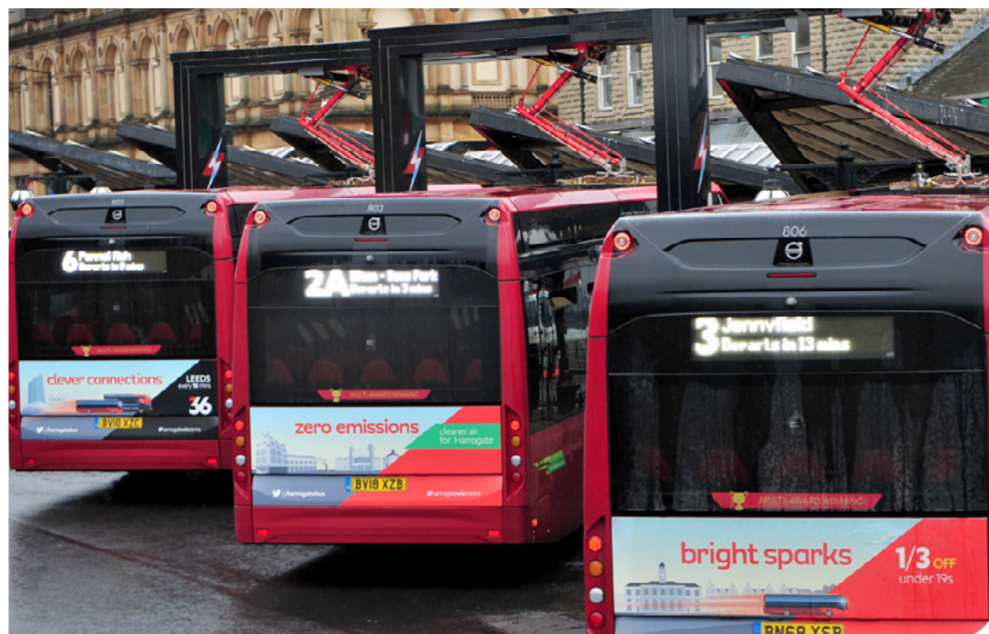
Figure 8: Opportunity on-route using conductive 'Pantograph-Down' charging system installed at bus stop.
