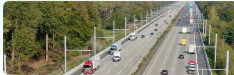
Catenary infrastructure on A5 in Germany (Image source: Hessen Mobil)
